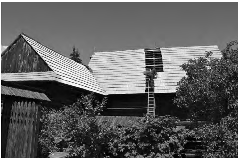
Fig. 4, 5. Placing a new shingle roof on the roof of the farmstead from Novot' and the residential house of the farmstead from Hruštín. Photograph by J. Neplech, 2018
